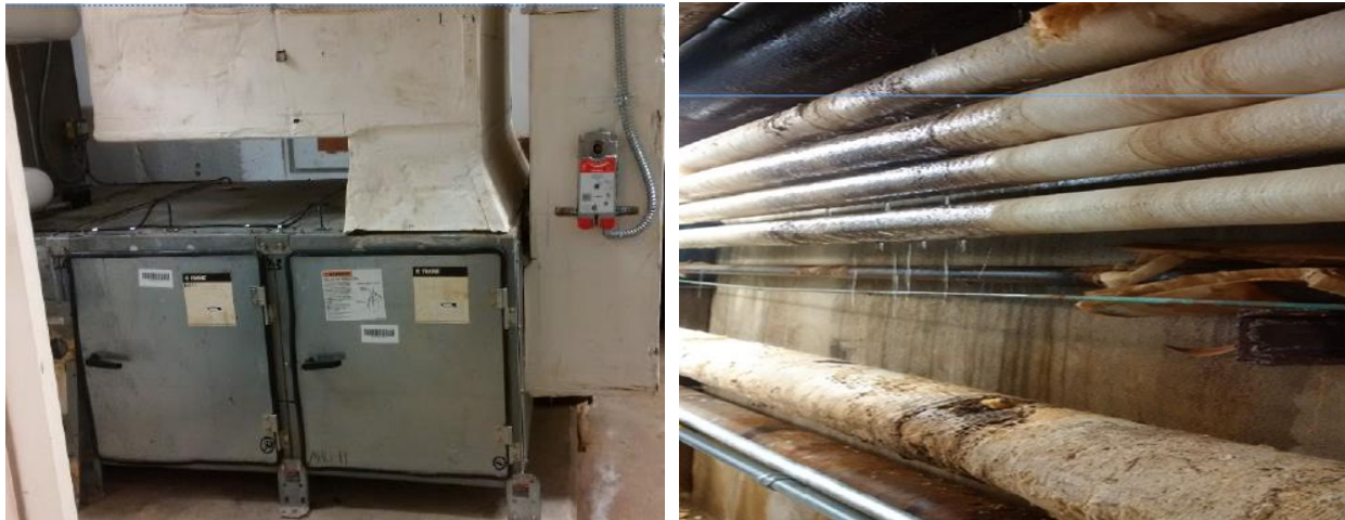
Figure 2. Eccles Air Handling Units Several Years Beyond Their Useful Life and Original, Abandoned Pipes with Dripping Water
